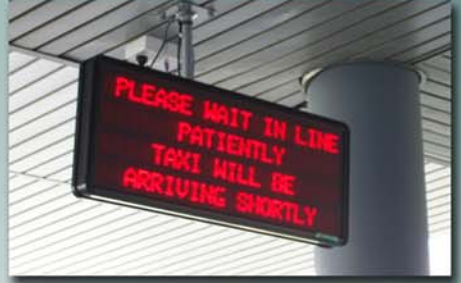
7. Perth Airport Taxi Queuing System
